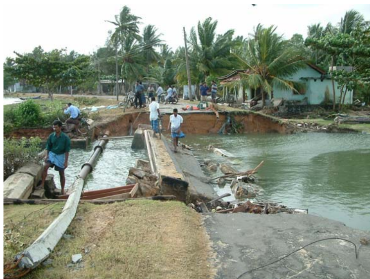
Damaged bridge in Ampara District
